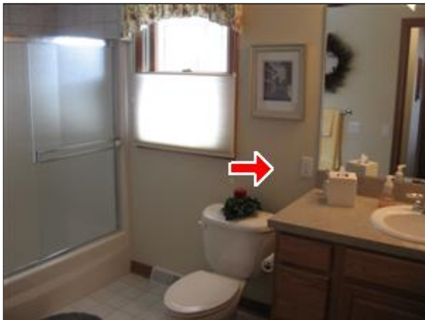
6.5.A Picture 1 GFCI in main floor full bath
