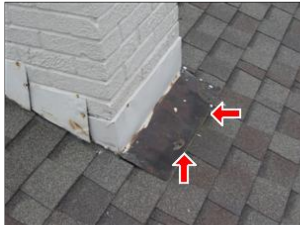
1.1 Picture 2 rusted thru flashin
