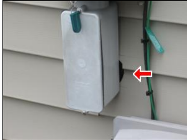
2.8 Picture 1 electrical service entrance
