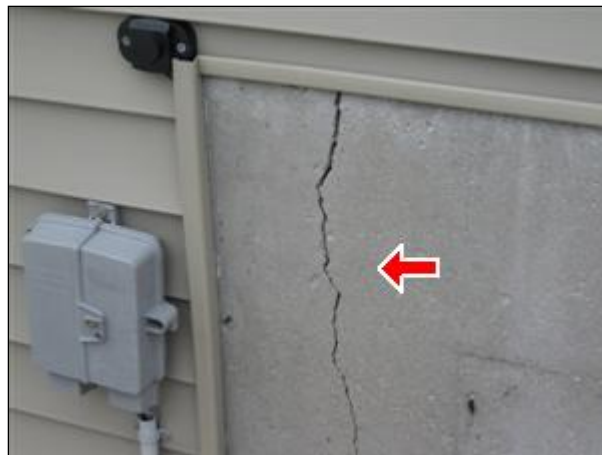
2.8 Picture 2 crack in foundation on North side of garage
