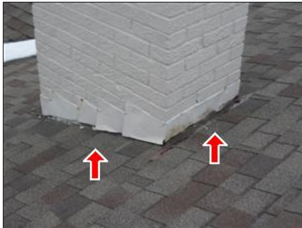
1.1 Picture 1 rusted and loose flashing
